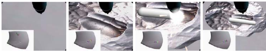
(a) Search the damaged area (b) Measure the flaw and programming (c) Repairing weld (d) Measure the welded area
