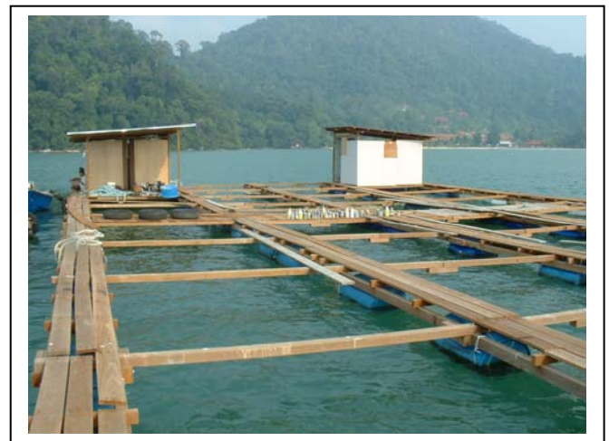
Figure 1. Tropical fish farm in construction phase. Each compartment is an individual fish cage.
