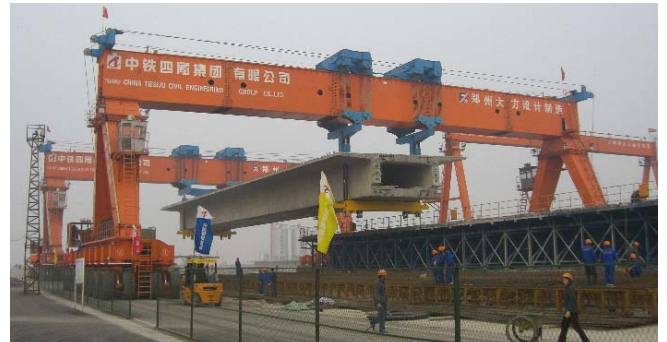
Figure 4. Working status of twin hoisting-girder transporters
