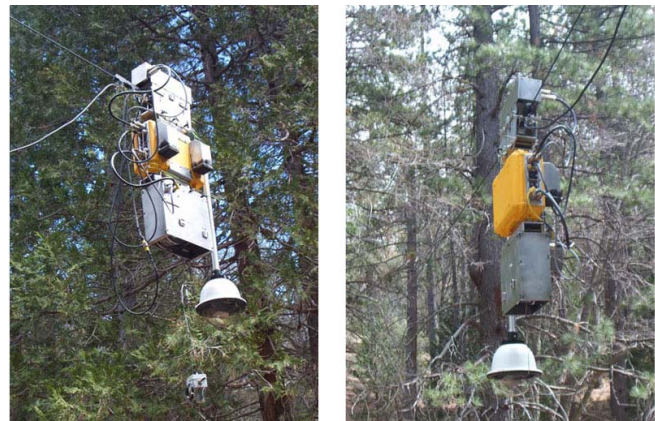
Fig. 1. NIMS systems developed for permanent installation in large scale forest environments. Although effective this system is not adapted to the new generation of rapid deployment applications that appear in addition to permanent deployment applications.
