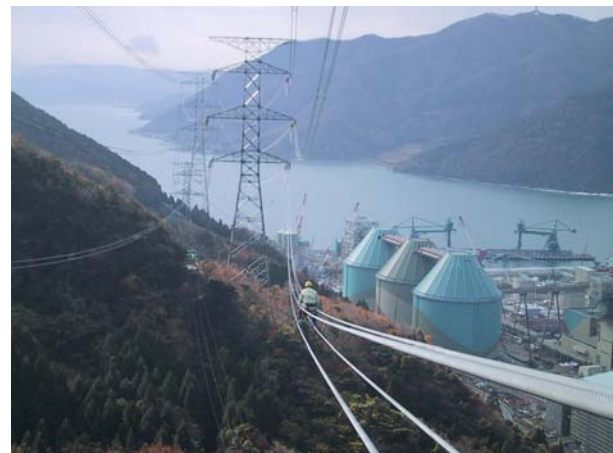
Fig. 1. Worker performing preventive maintenance on transmission lines, suspended tens of meters above the ground.
