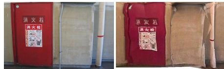
(c) Fire Hydrant
