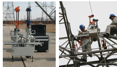
Fig. 2 AApe-B inspection robot and field performance tests.
