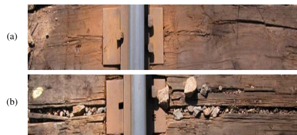
Figure 1. Wooden railway sleepers in different conditions, (a) Wooden sleeper in good condition. (b) A wooden railway sleeper in bad condition
