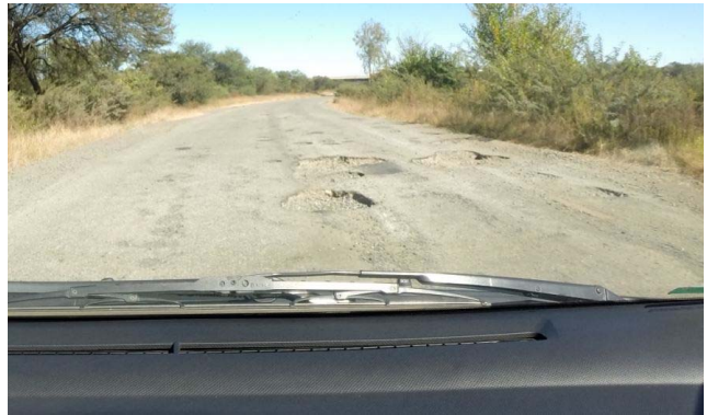
Fig. 1. Example of potholes in a road
