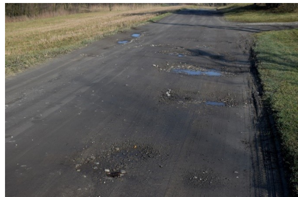
Fig. 1. Example of the potholes on a dirt road.
