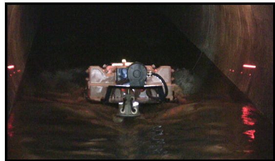
Figure 1: The cable-guided damage surveying system within a sewer pipe.
