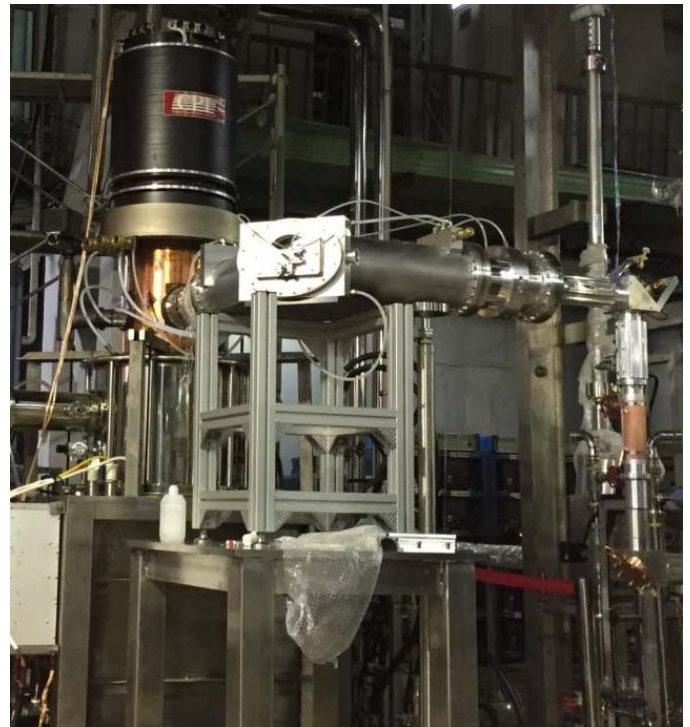
Fig. 3. Installation of the 140 GHz VGT-8141 SN2 Gyrotron at the ECH facility for the EAST tokamak. A single-mirror "elbow" matching unit focuses the output beam onto the aperture of the facility's transmission line system.
